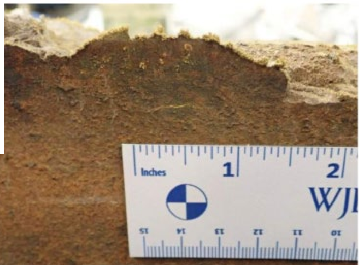
Figure 2. Crack highlighted by yellow filings in 1 3/8-inch thick plate at fracture.
