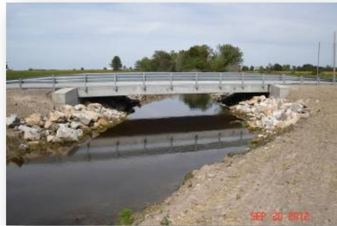
Audrain County, MO Bridge 336 Built 2012 Precast 6 Hollowcore Slab Girders 50.5 ft. Span 24 ft. Roadway Width 2 ft. Structural Depth 20° Skew
